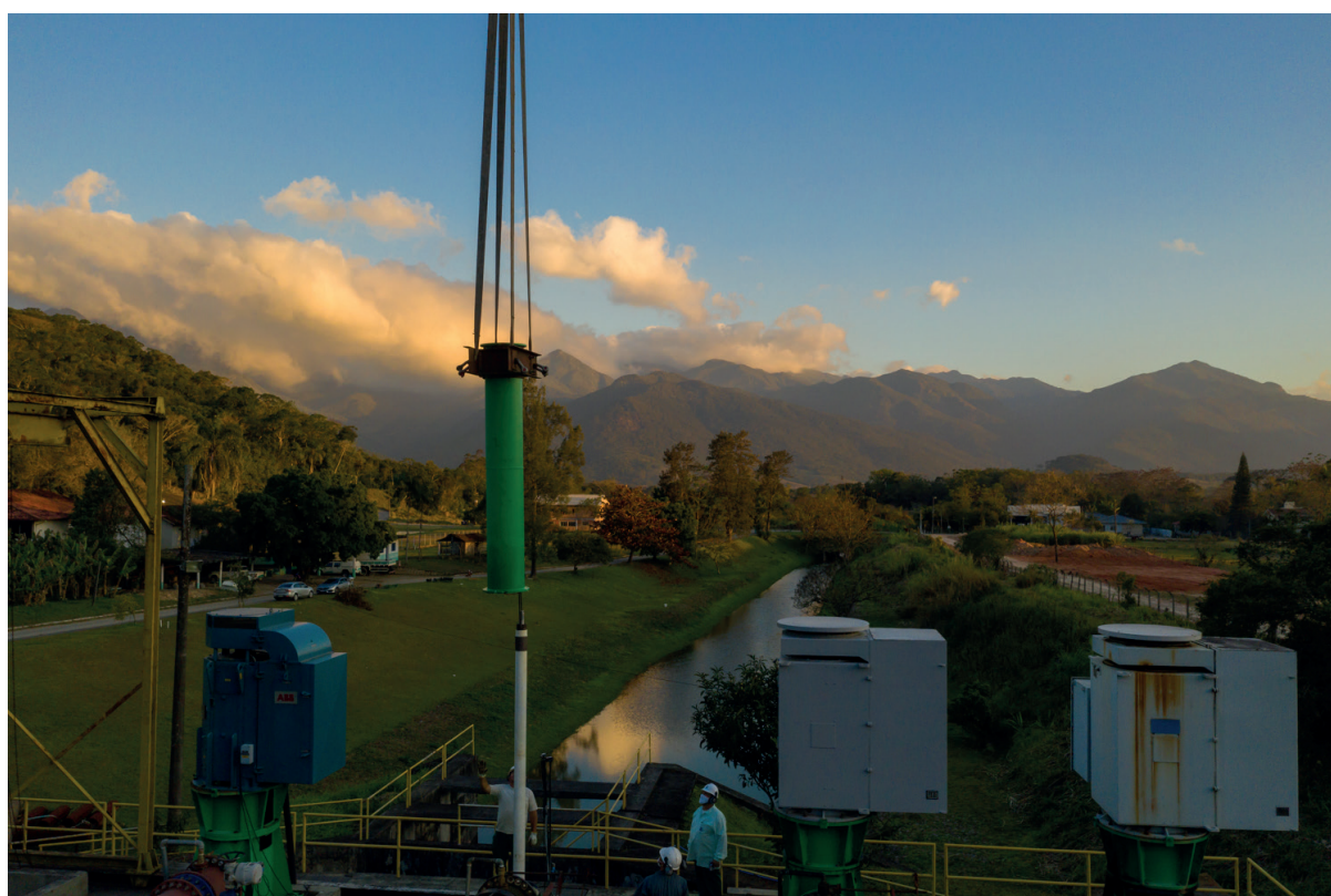
Image: Infrastructure for expanding water collection in the Cubatão River. Source: CASAN website.
